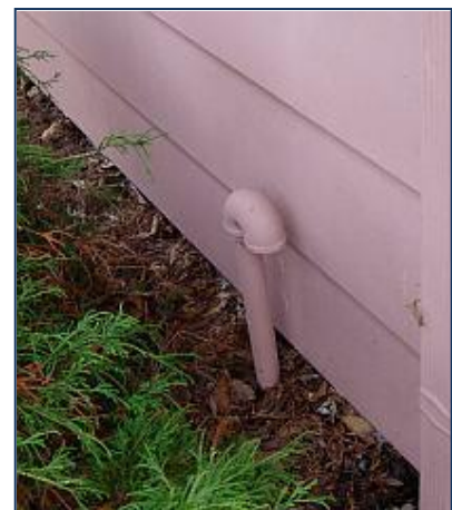
A vent for an underground storage tank is an indication that the tank is still present.
